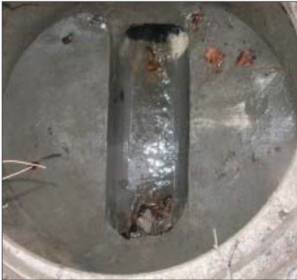
The manhole floor is renovated with a new channel and the berms are subsequently re-cast.
