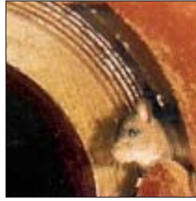
Rats find nesting places in unused and defective laterals.
